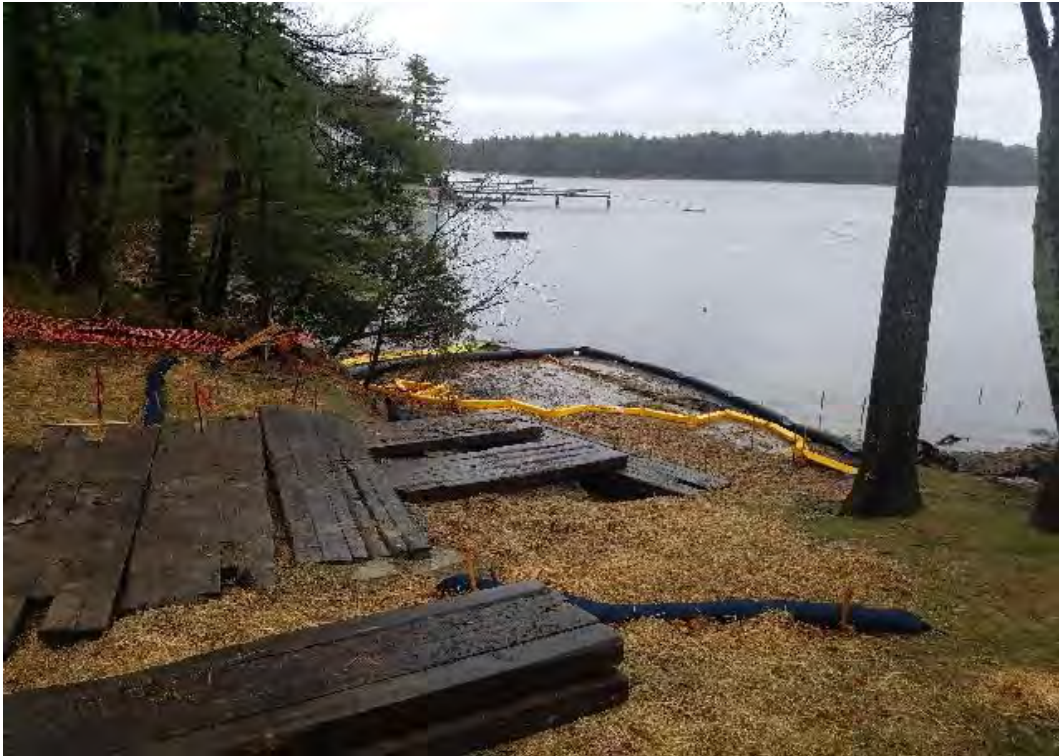
Fig 3: Installing timber mat access road below manhole at Gundalow landing. Viewing south. (04-27-20).
