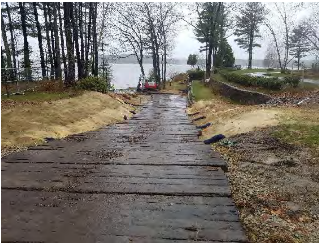
Fig 2: Continuing to install timber mat access road at Gundalow landing/east side of the Bay. Viewing southwest. (04-27-20).
