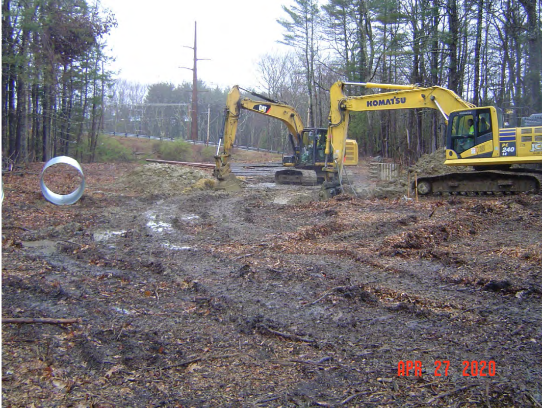
Fig 5: Hammering ledge at Str. 33. Viewing northeast. (04-27-20).
