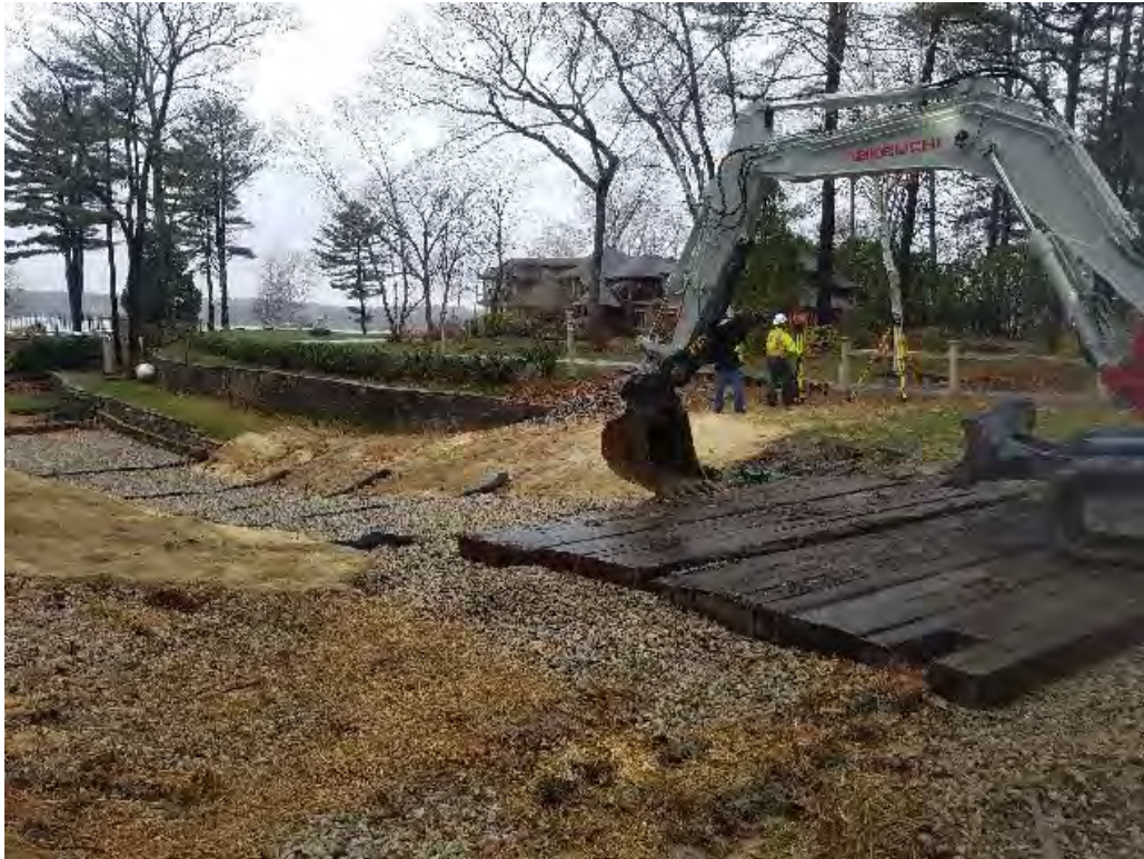
Fig 1: Installing timber mat access road at Gundalow landing/east side of the Bay. Viewing west. (04-27-20).
